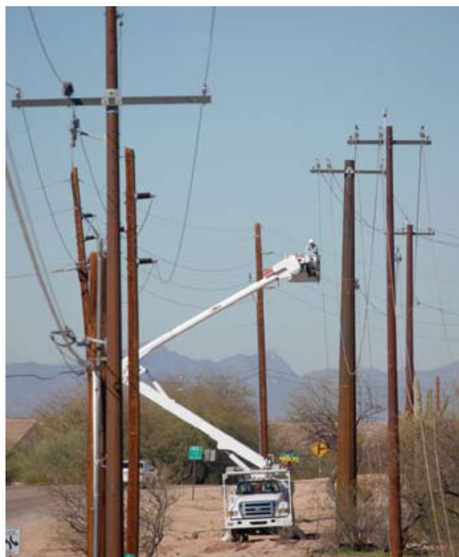
Crews relocate a line because of a road improvement project and use steel for the new poles.
