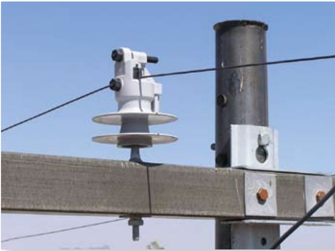
Hendrix polymer vise-top center-phase insulator (shown prior to the raptor hood being installed) is the Tucson Electric Power standard.
