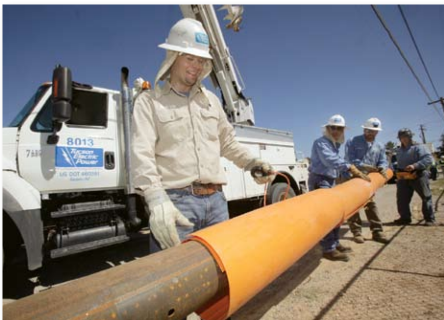
Crew installs cover-up over the steel to provide protection in case of accidental contact with an energized line.
